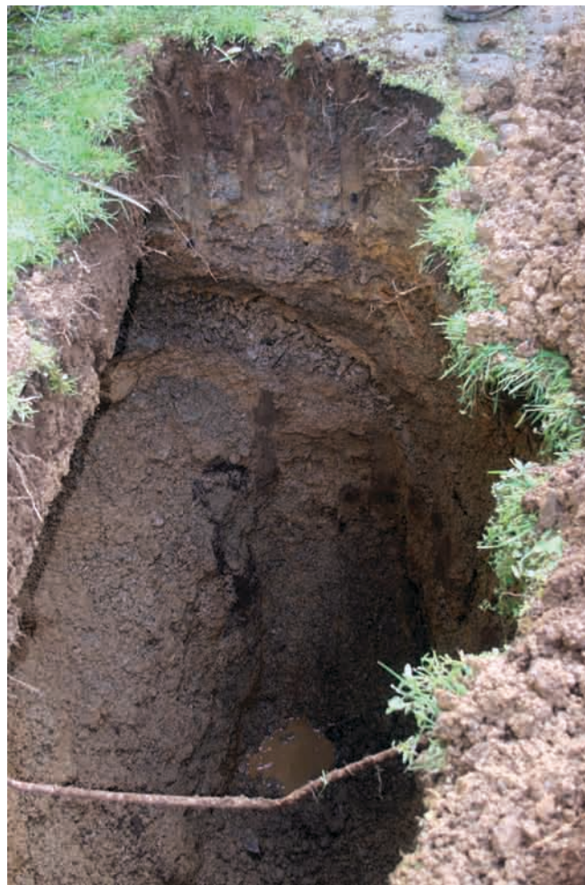
Figure 1. Test Pit 1 showing layers of reclamation fill in the end wall. The reclamation fill beneath the north wall (right) has collapsed away.
